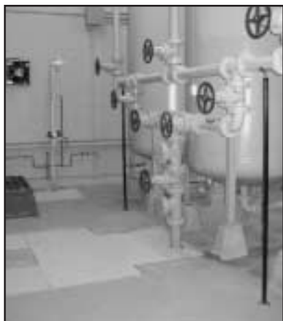
Tanks inside the new plant
