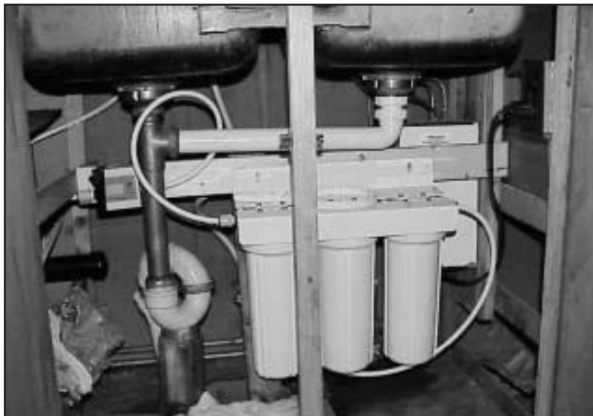
POU (Point of Use) filter cartridges for the treatment of Arsenic in a residential area.
