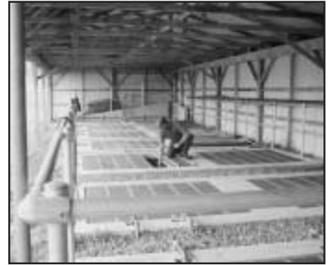
The current, small, activated sludge treatment plant, Farmington
