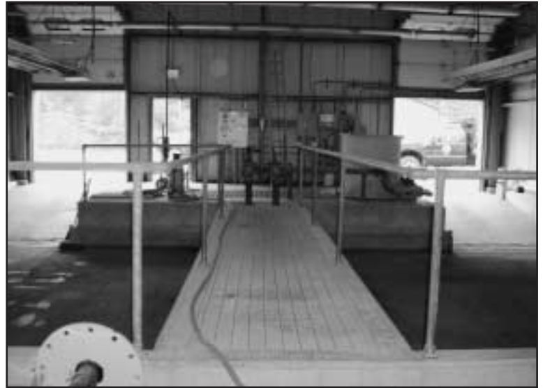
The dual drying beds have never worked properly
