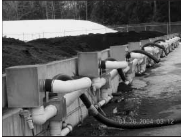
Close-up of blowers for aerating compost
