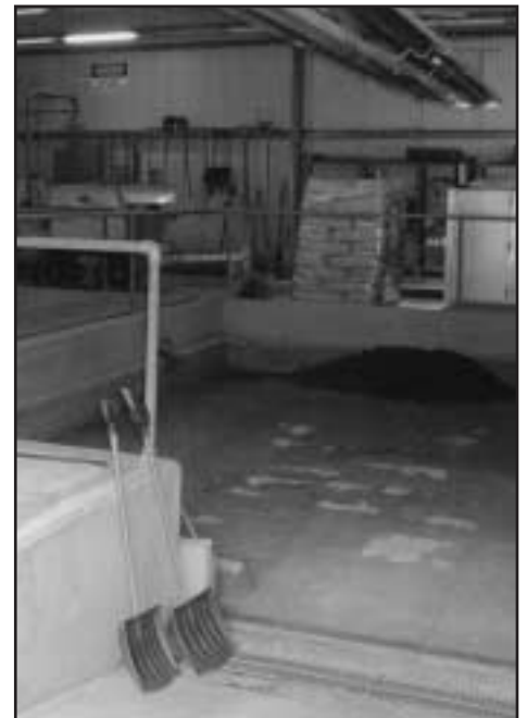
The belt filter press will eliminate the need for the operators to manually shovel sludge
