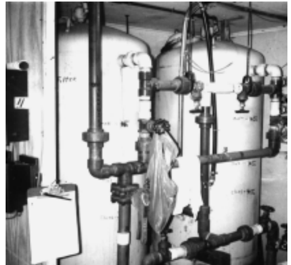
Coaldale had to replace filters: Green sand filters remove iron and manganese from drinking water. This filtration is commonly used throughout PA in areas previously subjected to coal mining.
