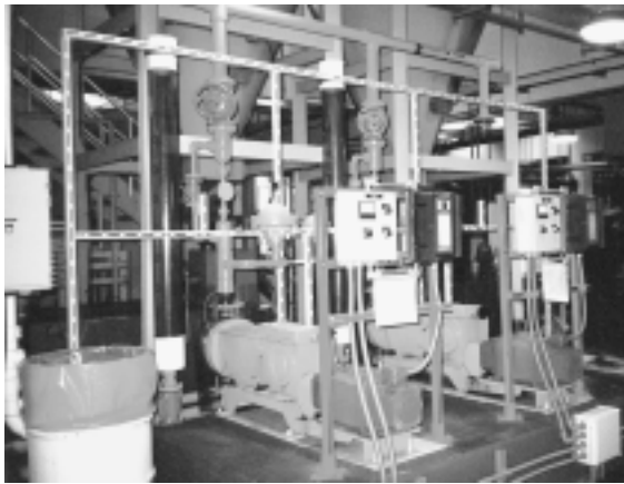
Chemical processing area, drinking water treatment facility
